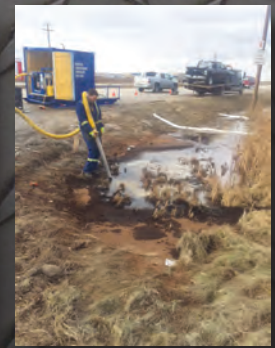
Diesel spill vac cleanup
